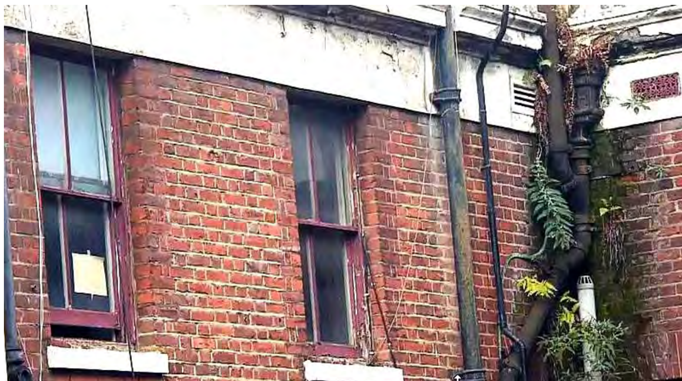
Many parts of the Victorian hospital are showing signs of disrepair
